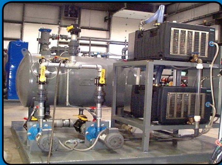
AIRVAC 1,000 gallon vacuum collection station with dual vacuum and discharge pumps.
