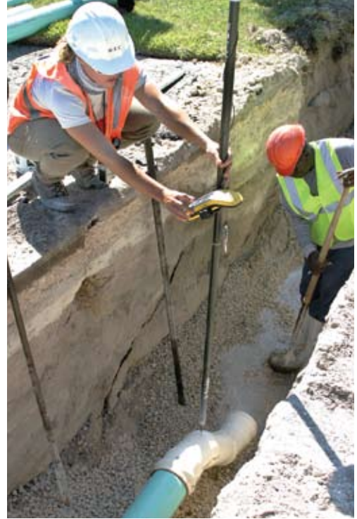
For future reference, crews mapped the vacuum collection lines and valve pits precisely with GPS technology.
