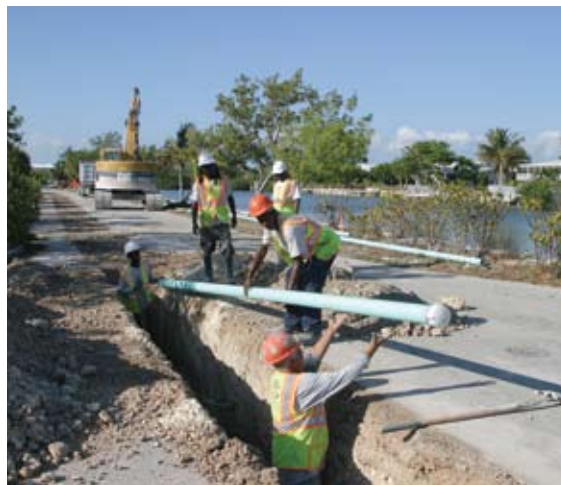
Shallow trenches and lightweight PVC pipe made installation of a vacuum sewer system fast and less disruptive to residents and tourists.
