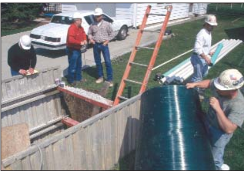
Contractor, engineer and municipality worked together to provide the citizens of Forest, OH, a state-of-the-art sewer system.
