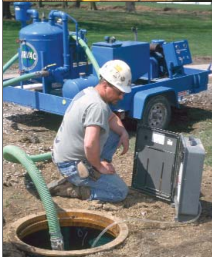
Top: Many vacuum sewer components can be installed by hand, saving equipment costs and reducing installation time. Here, two workmen lower a vacuum valve pit into place in a Forest, OH, neighborhood.
