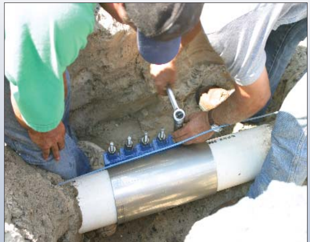
Repairing the damage was relatively simple, as the shallow depth of the line made access easy. A full-circle clamp was applied and the line was back in service in less than an hour.
