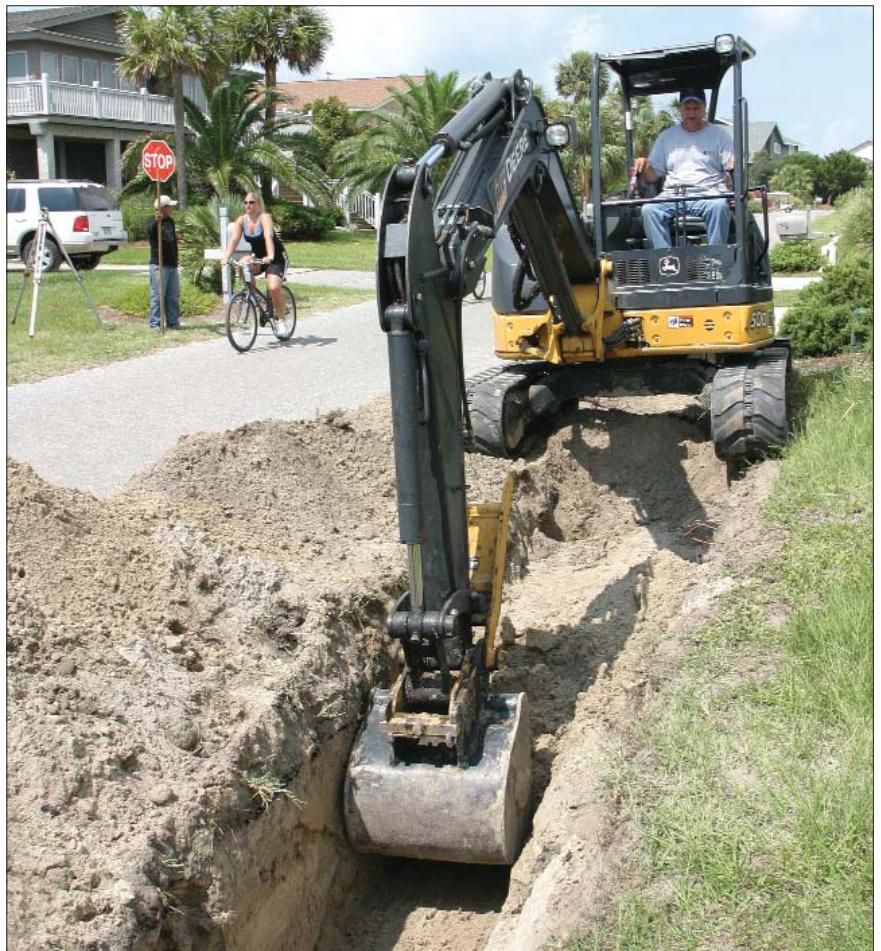
Vacuum sewers are typically buried in shallow trenches, so contractors can use smaller excavation equipment and there is less soil displacement, allowing streets to remain open.
