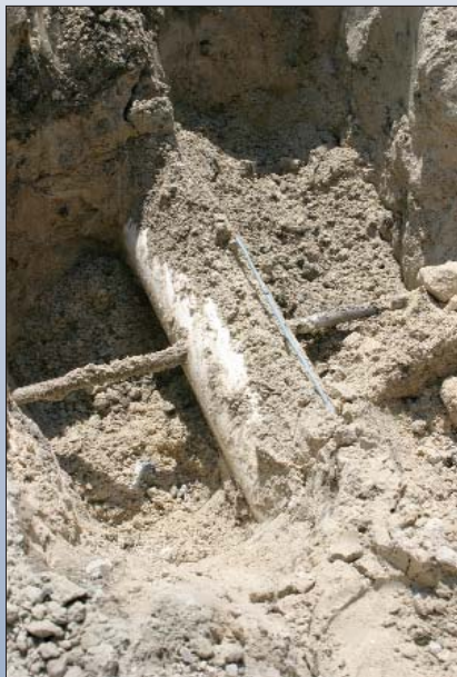
Workmen accidentally hit a Fripp Island vacuum sewer collection line dead center when installing cable.
