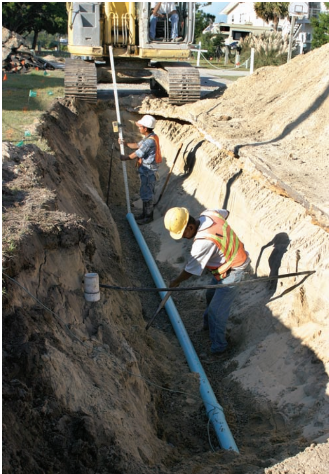
Lightweight, vacuum collection lines, typically 4 inches to 10 inches in diameter, can be buried in trenches only about 4 to 6 feet deep.
