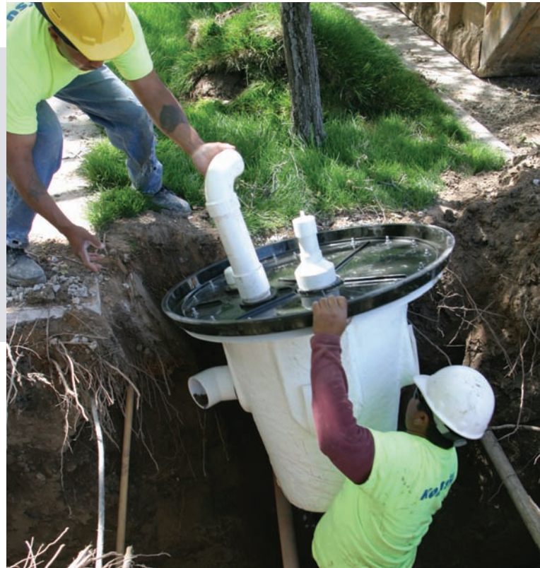
Hooper's vacuum sewer system, including valve pit sumps (shown here) was installed amid existing utilities with no disruption of service or inconvenience to residents.
