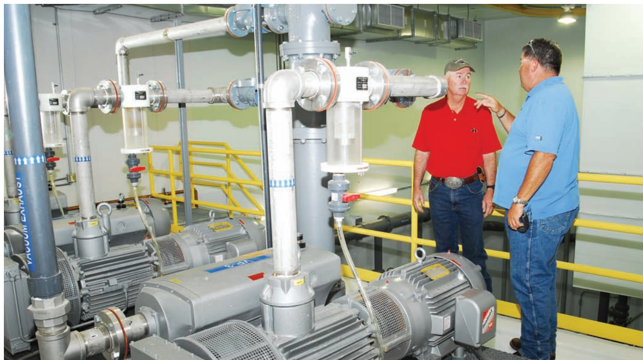
Sewer System Manager Dennis Steele (right) discusses operating details with Technician Tym Fowers inside one of Hooper’s new vacuum stations.
