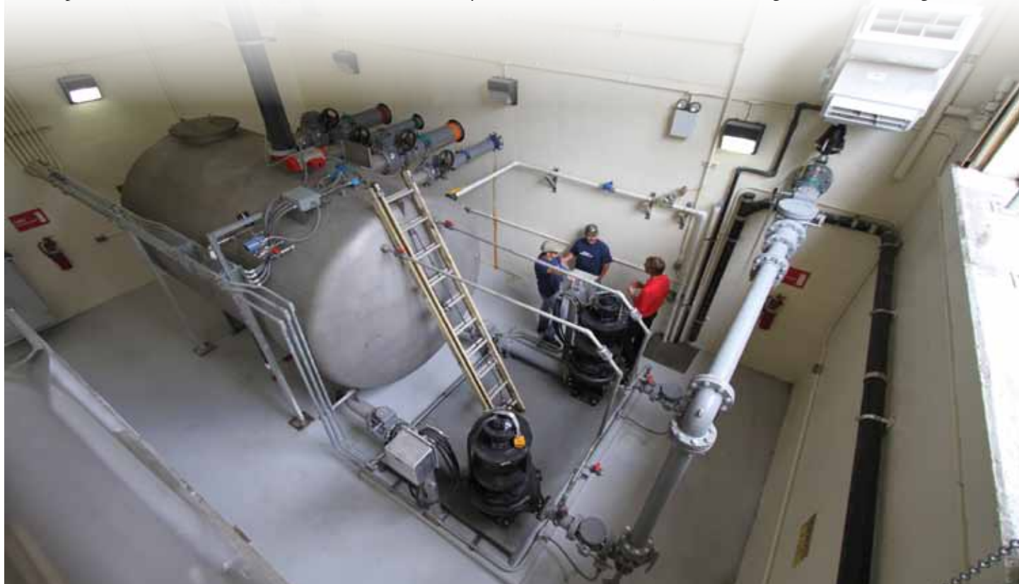
Vacuum sewer stations are clean, odor-free working environments that cover a relatively small footprint. They can be located in residential neighborhoods and designed to blend in with local architecture.
