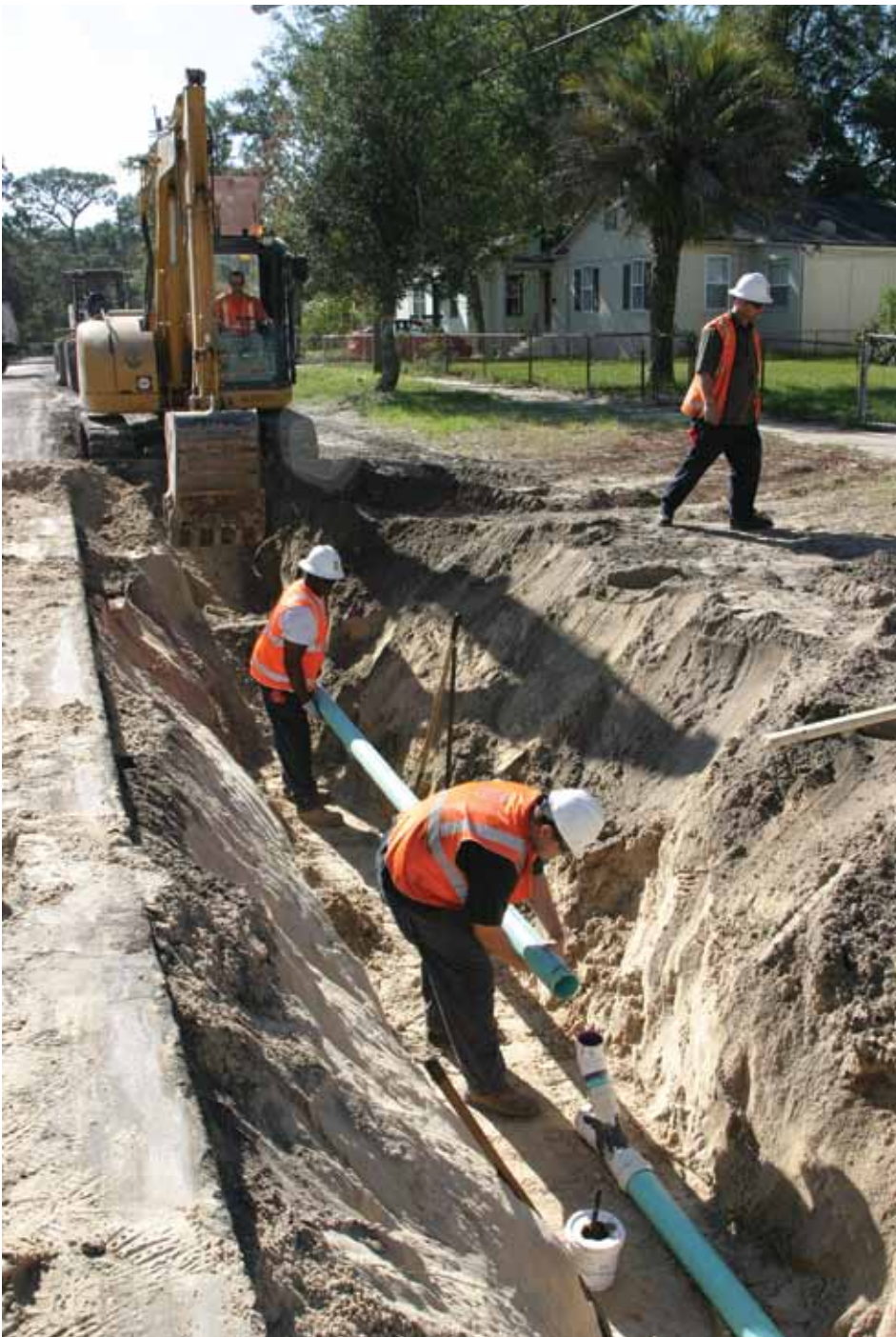
Vacuum sewer mains require shallower trenches than most gravity sewer lines, so there is less disruption, less equipment and faster, easier installation.
