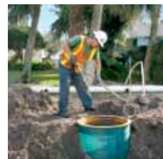
One valve pit can serve several homes.
