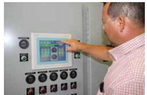
Monitoring the pressure levels at JEA’s modern vacuum sewer station takes only a few minutes each day.
