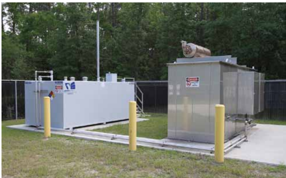
A reserve generator (right) and diesel supply are ready to power the vacuum station if there is ever a loss of electrical power.
