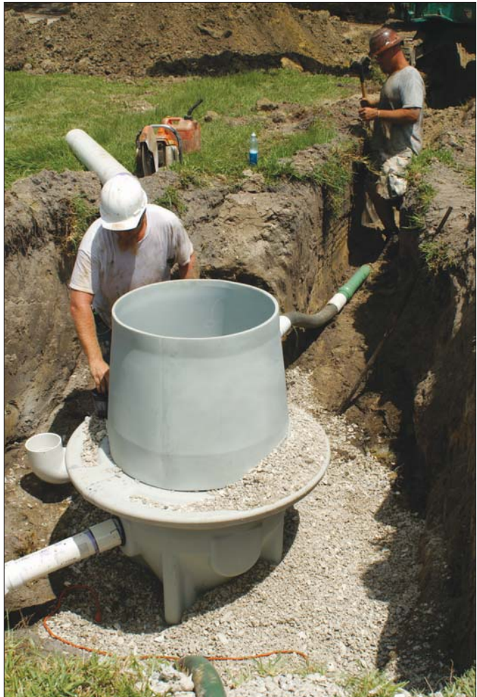
Shallow installation of vacuum sewer pits was important in Rockridge because the community is located on a layer of rock covered by sandy soil—making deep excavation costly—and in addition, groundwater levels are high.
