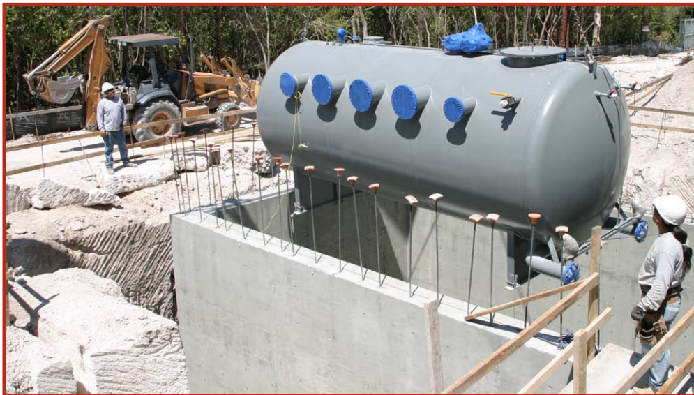
A prefabricated sewage collection tank is lowered by crane into an AIRVAC vacuum sewer station in Key Largo, Fla.
