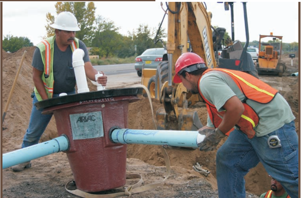
An AIRVAC valve pit operates pneumatically, no electricity is required. When the wastewater reaches a predetermined amount, it discharges into the vacuum main and sent to the vacuum station. (Albuquerque, NM installation)
