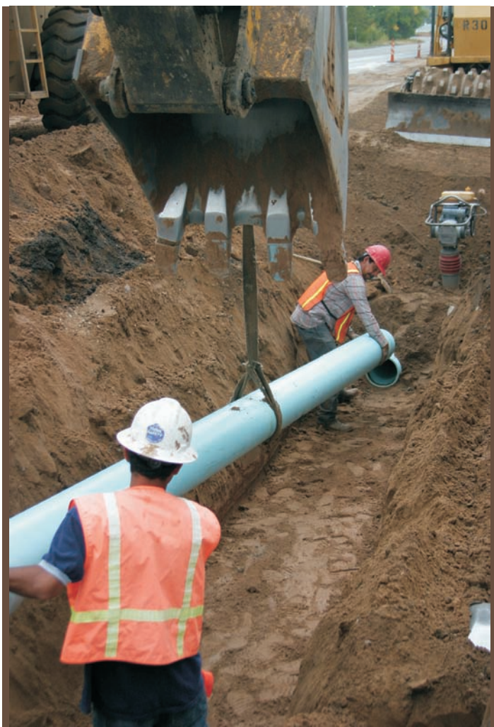
Shallow trenches and lightweight PVC pipe make installation fast and less disruptive.
