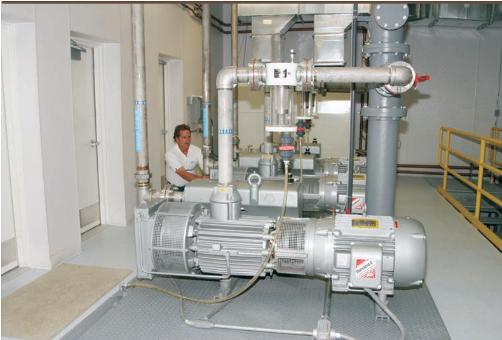
Negative pressure in the collection line is maintained by vacuum pumps located at the vacuum station.
